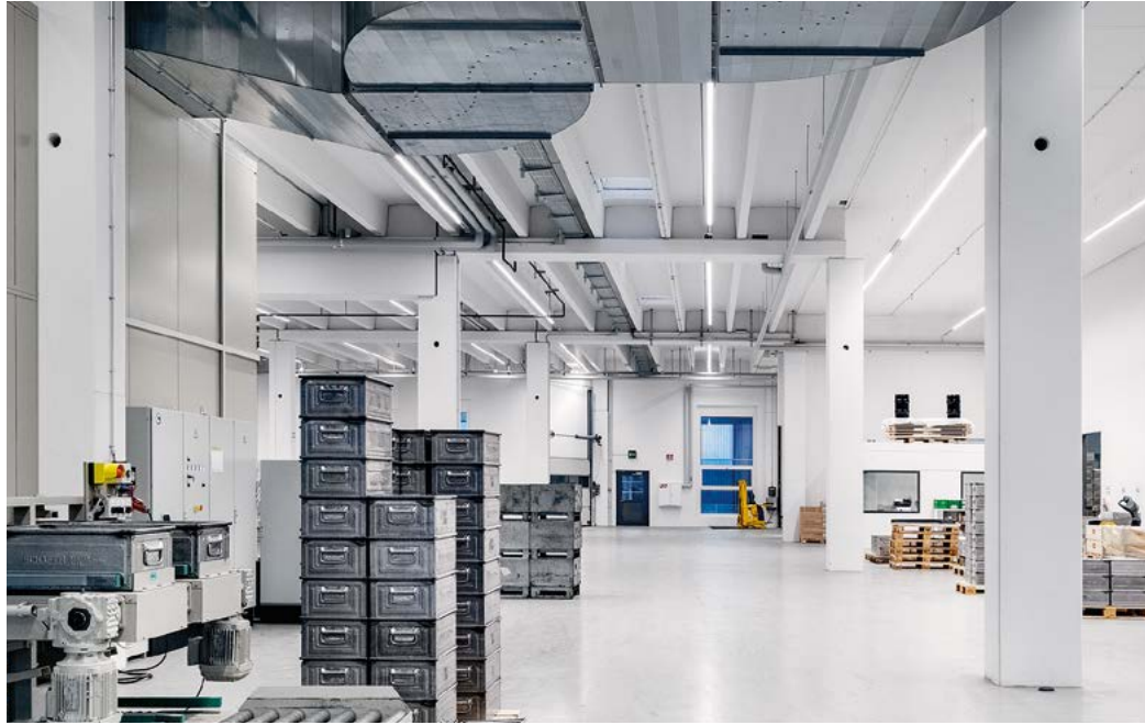
Galvanising plant, Kriessern | CH
